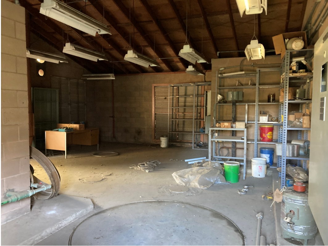
Interior of the chlorination structure, view from the main door
