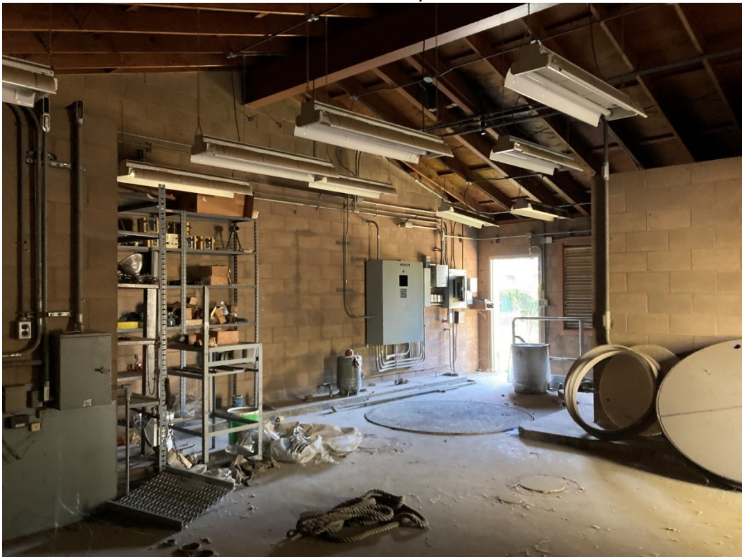
Interior of chlorination structure, view towards front door
