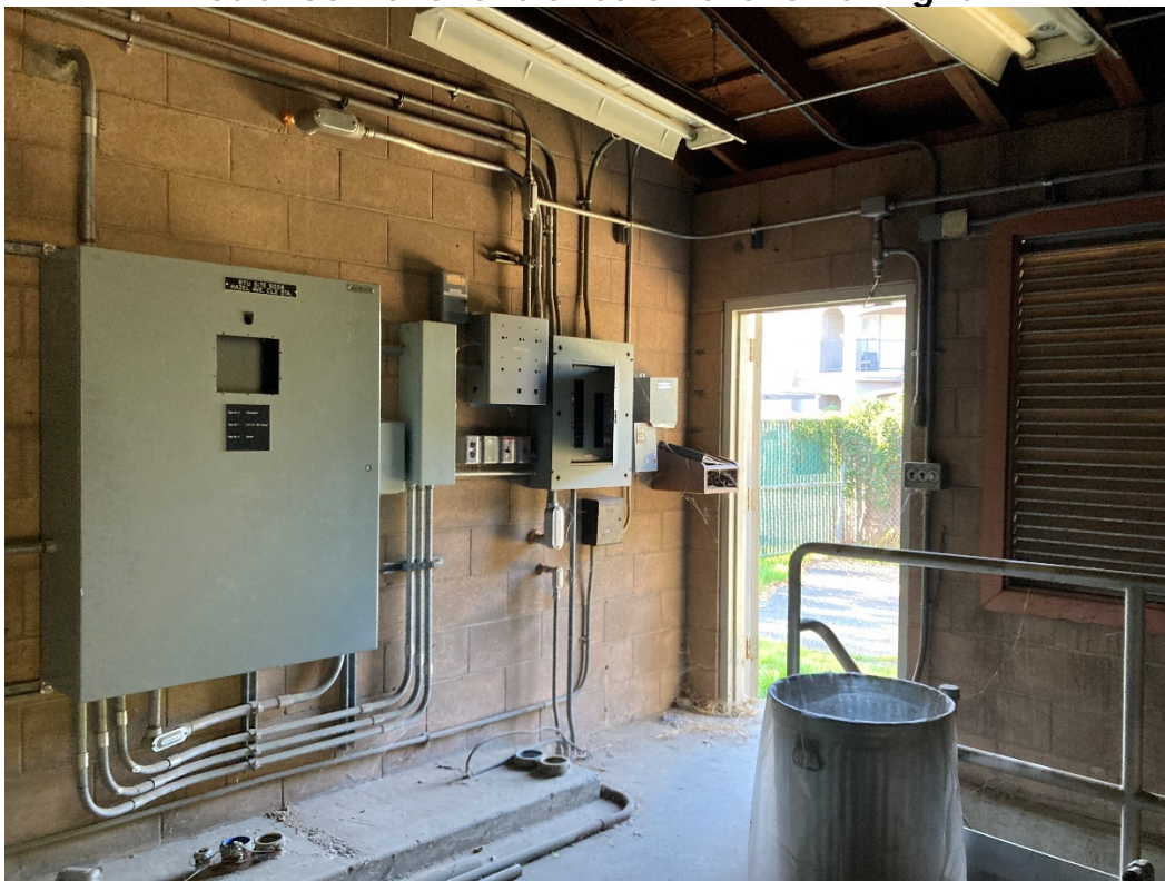
Interior of the chlorination structure, view towards the front door, subfloor level entrance on the lower right
