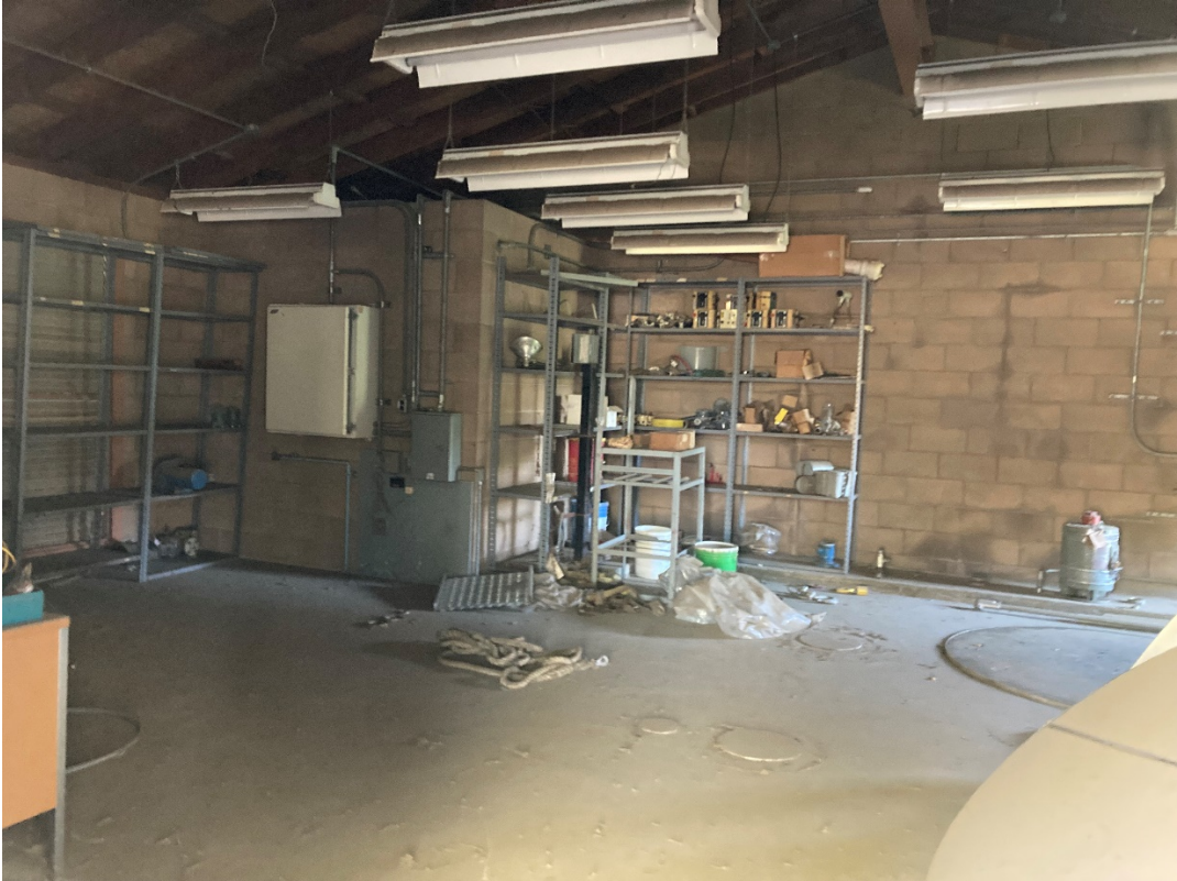
Interior of the chlorination structure, view from back door
